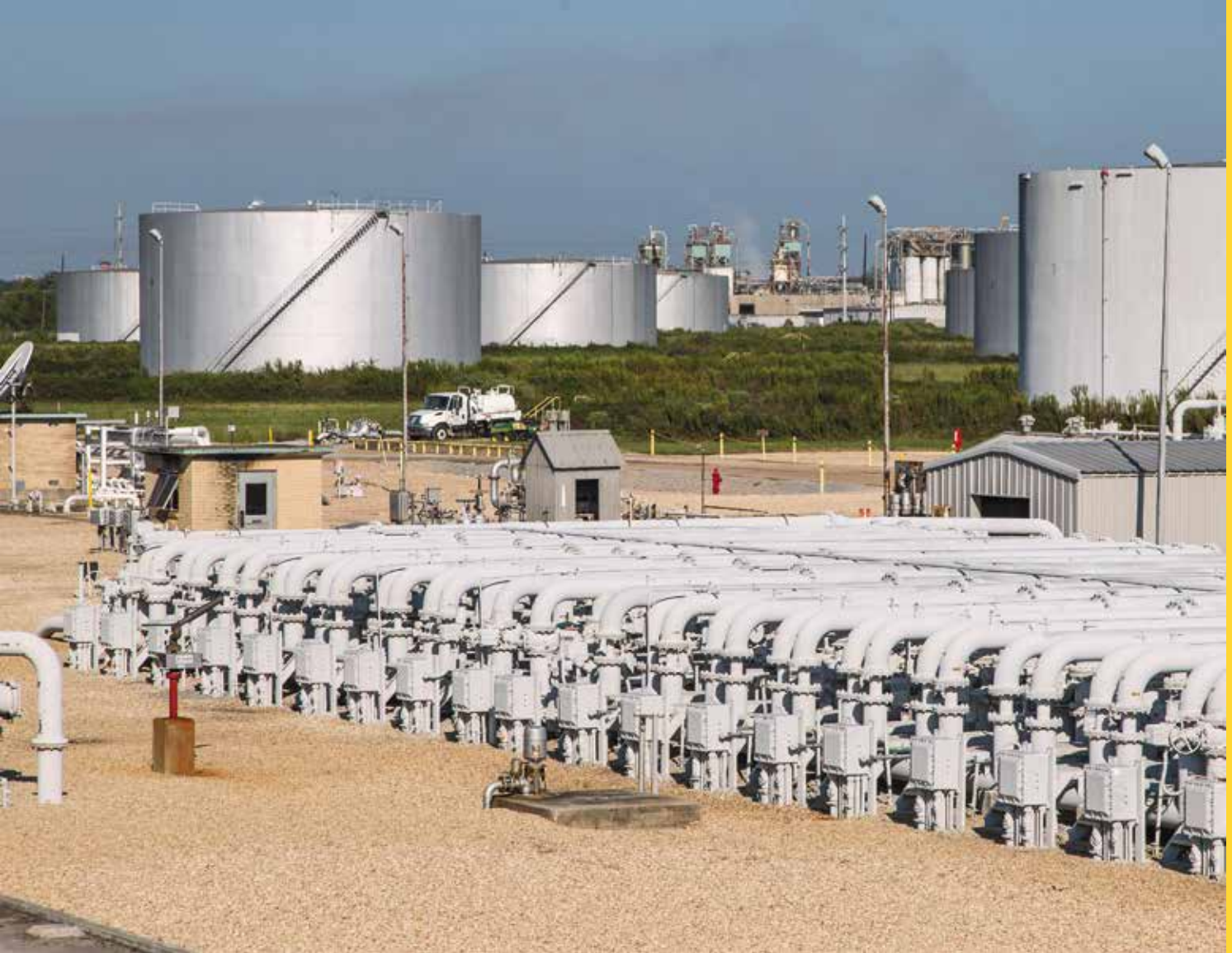
The Plantation Pipe Line Company operated by Kinder Morgan, 2015. Photo by LSU.
